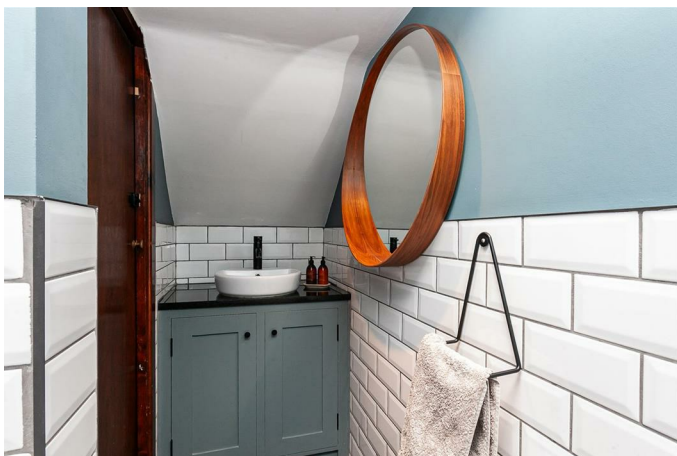
Low flush W.C, wash hand basin with vanity unit below, part tiled walls.
